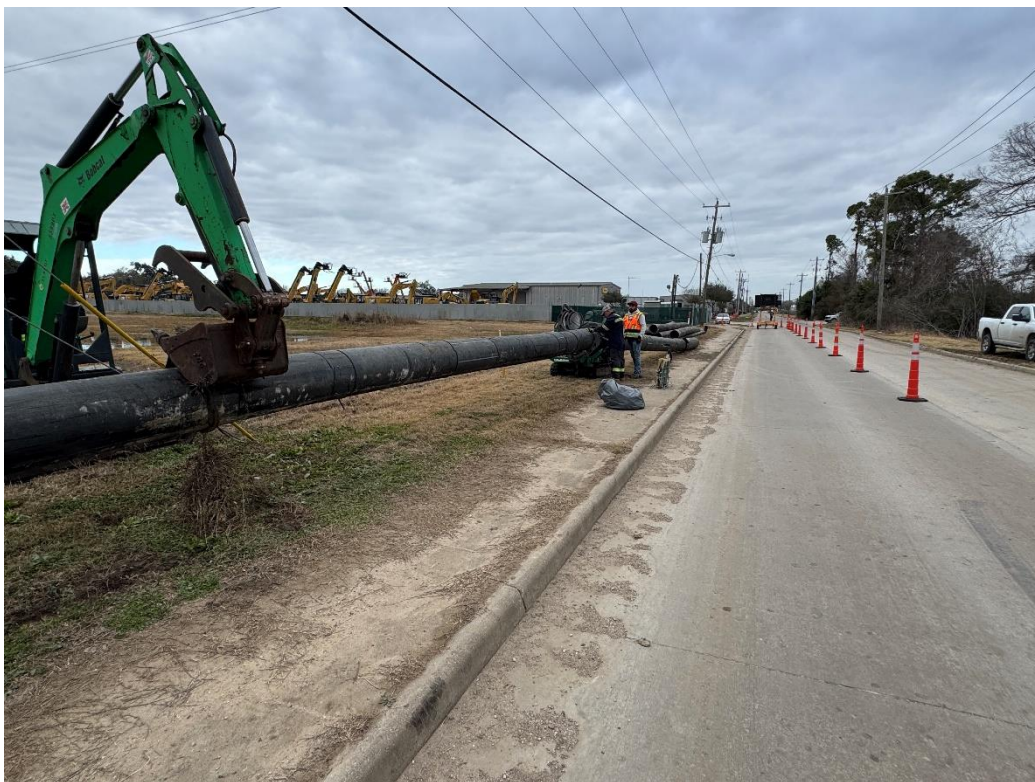
Bypass piping setup
