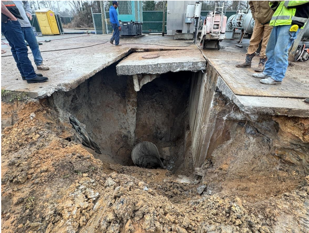
Failure of manhole and 42" gravity sewer into lift station
