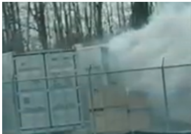
Figure 2: An ESS Fire in Standish, MI USA.
