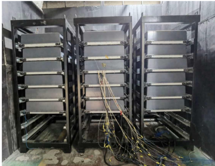
Figure 18: A picture of the test setup. This image was taken from the UL 9540A unit-level test report [8].
