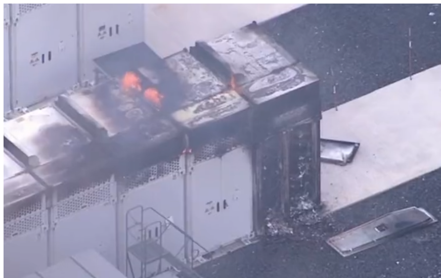
Figure 4: A fire in a Powin battery storage unit in Warwick, New York [22].
