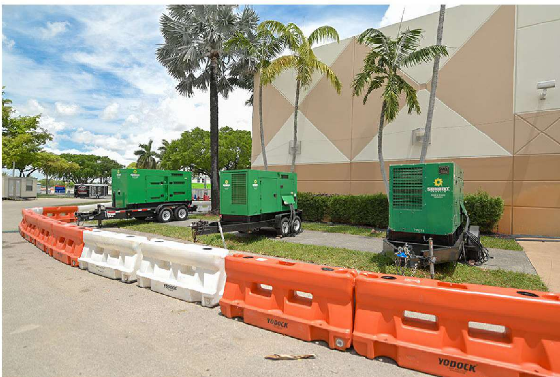
Deployed Generators in Support of Florida COVID-19 Response
