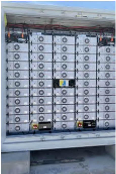
20ft x 8ft air-cooled enclosures
