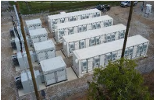
15x 9.9MW/11MWh BESS Largest Traded BESS Fleet 2020-2021 Broad Reach Power
