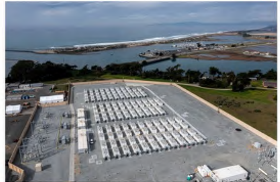
Batteries at a storage system in Moss Landing, California. Photographer: David Paul Morris/Bloomberg
