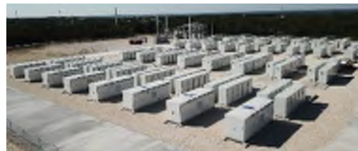
2x 100MW/110MWh BESS Former Largest BESS in Texas 2021 Broad Reach Power
