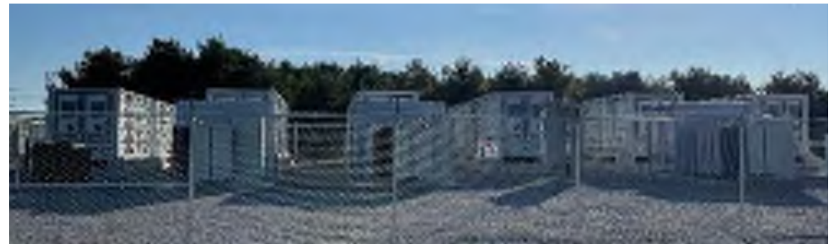
5x 6MW/21MWh BESS Time of Day Shifting BESS 2021-2022 Midwest REMC
