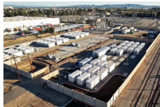
537MW/2414 MWh BESS World's largest BESS program 2021-2022 Southern California Edison
